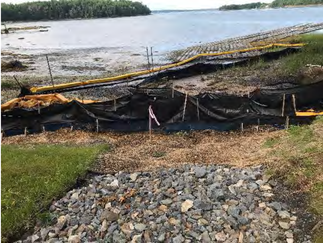
Fig 15: Toe of slope below manhole at Gundalow Landing/east side of the bay. Viewing southwest. (08-05-20).
