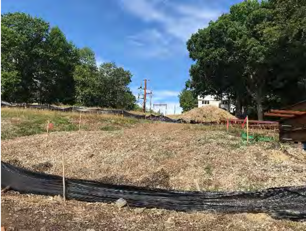
Fig 19: Slope above salt marsh restoration at Eversource property/west side of the bay. Planned final location of the cable house marked with orange flagged stakes. Viewing west. (08-03-20).
