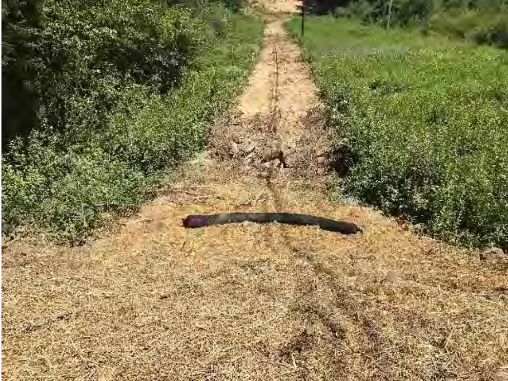
Fig 9: Timber mats removed from access road across wetland DW31. Wetland and slope down into wetland seeded and mulched. Silt sock BMP place in preparation for potential storm event. Viewing northeast. (08-03-20).
