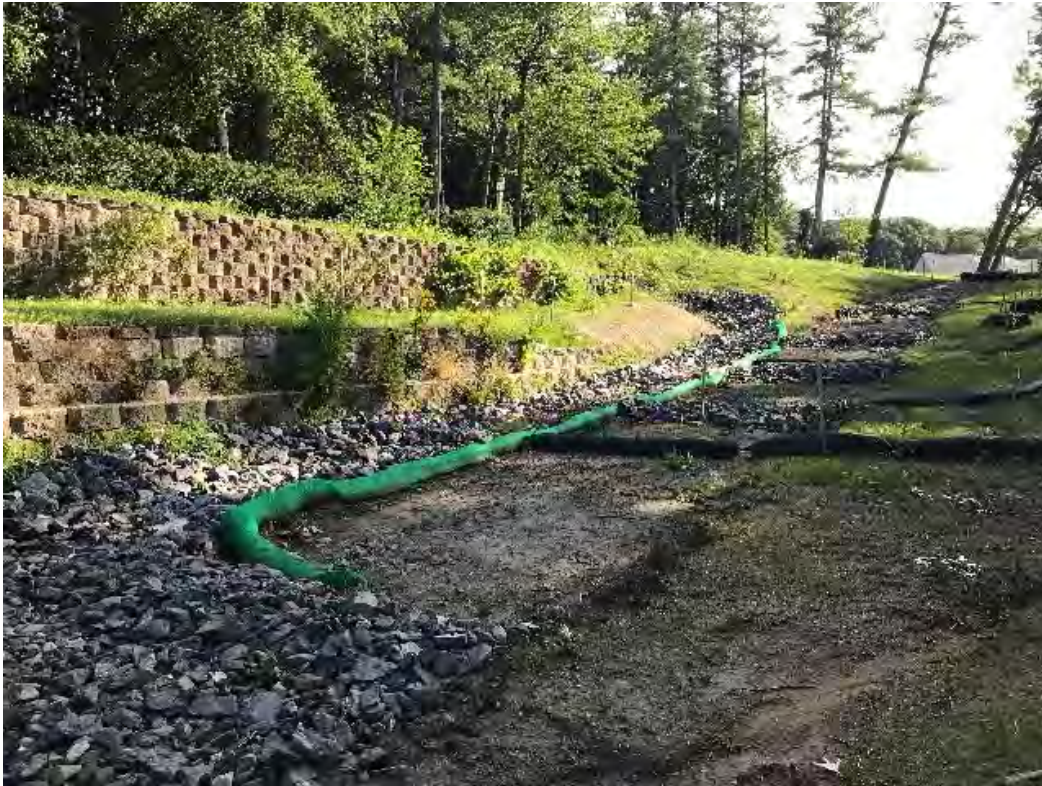
Fig 17: Slope above the manhole at Gundalow Landing/east side of the bay. Viewing northeast. (08-05-20).
