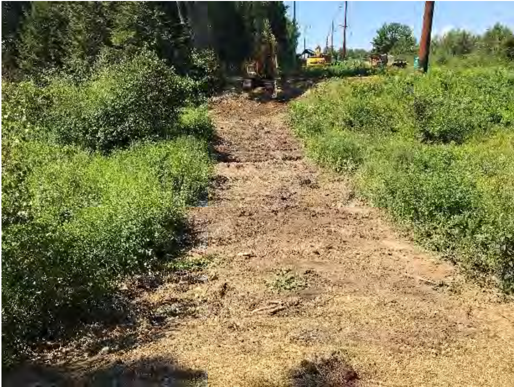
Fig 13: Timber mat removal and access road restoration at DS46 stream crossing. Viewing southwest. (08-05-20).
