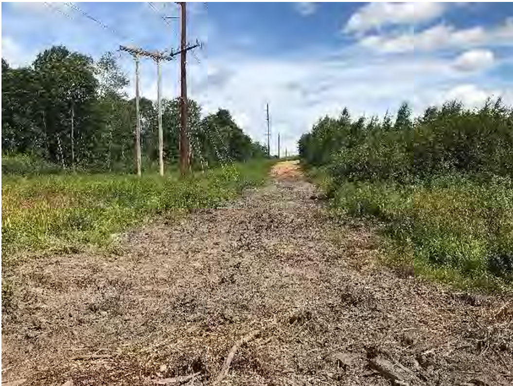
Fig 2: Access road across DW56, between Strs. 47 and 48. Timber mats removed and wetland seeded. Viewing north. (08-03-20).
