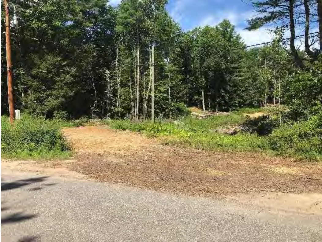
Fig 1: Culvert replacement in access road to Str. 93 off Durham Point Rd. complete. Seeded and lightly mulched. Viewing west. (08-03-20).
